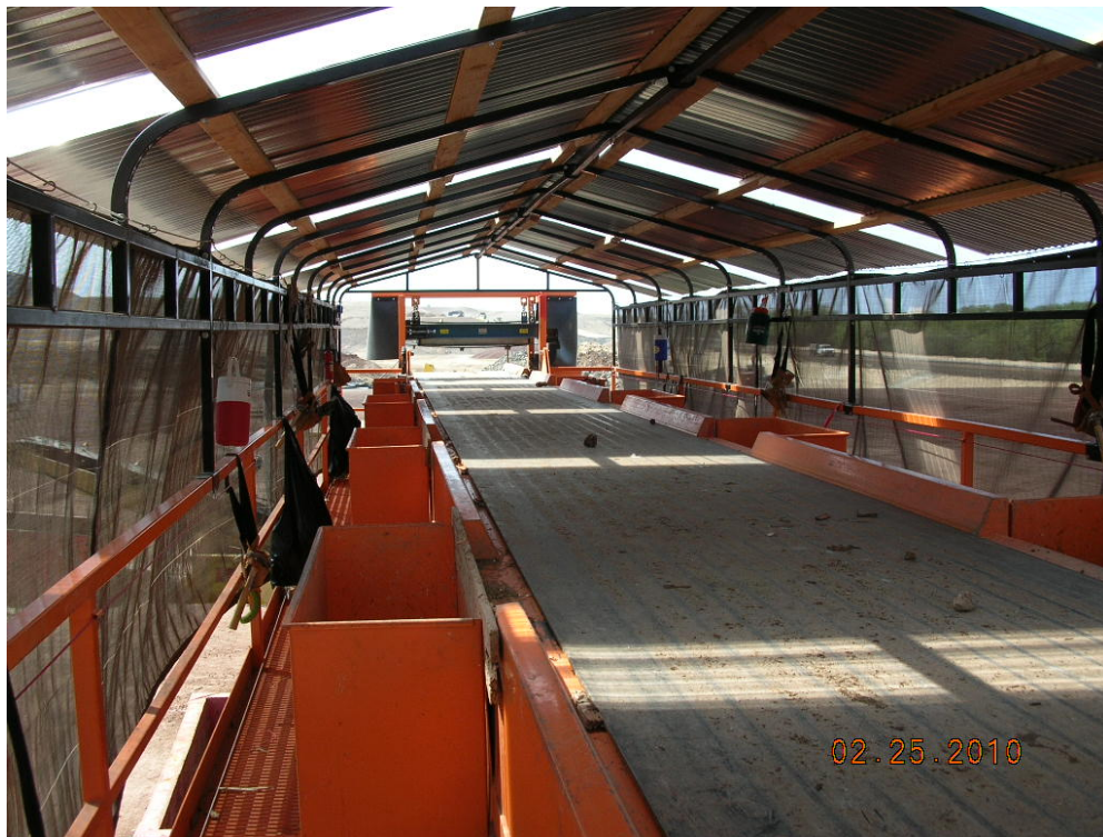
Conveyor Belt to Chipper
