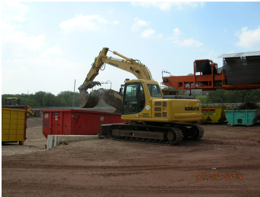
Chipper Collection at Rolloff Bin
